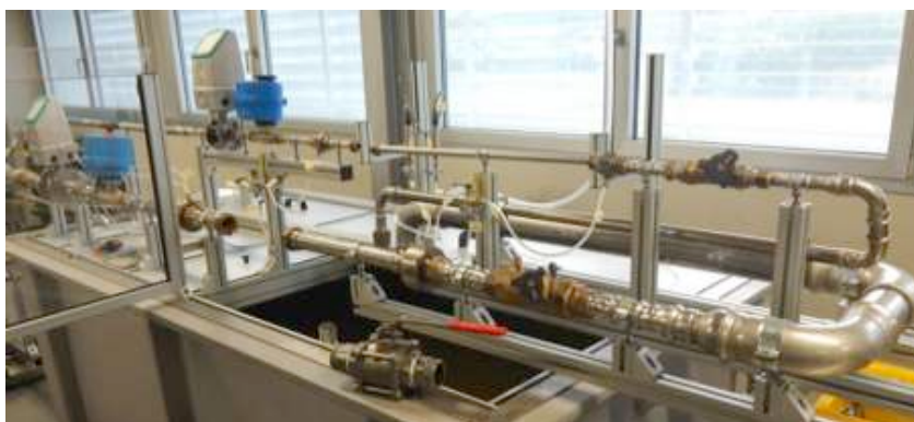
Rubinetterie Bresciane – Flow Loop testing facility
